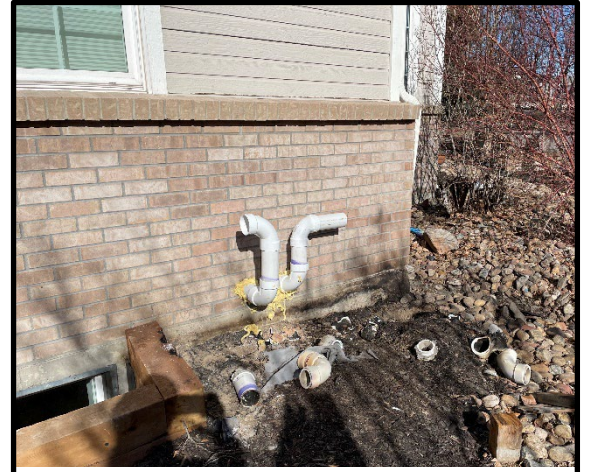
No protection on vents
