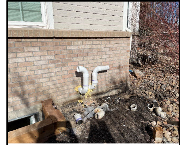
No protection on vents
