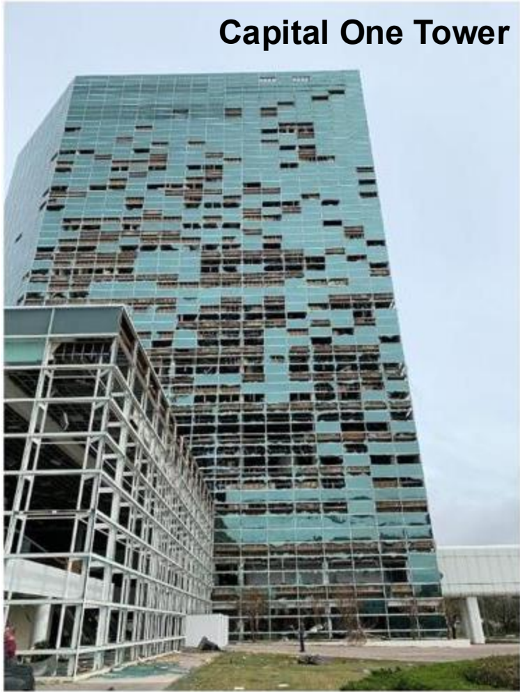
Building façade damaged by windborne debris in Hurricane Laura in 2020
