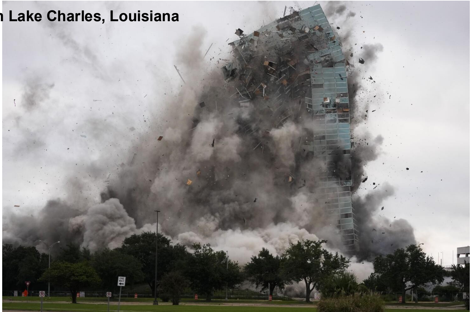
Building demolished by on September 7, 2024, because it is too expensive to repair
